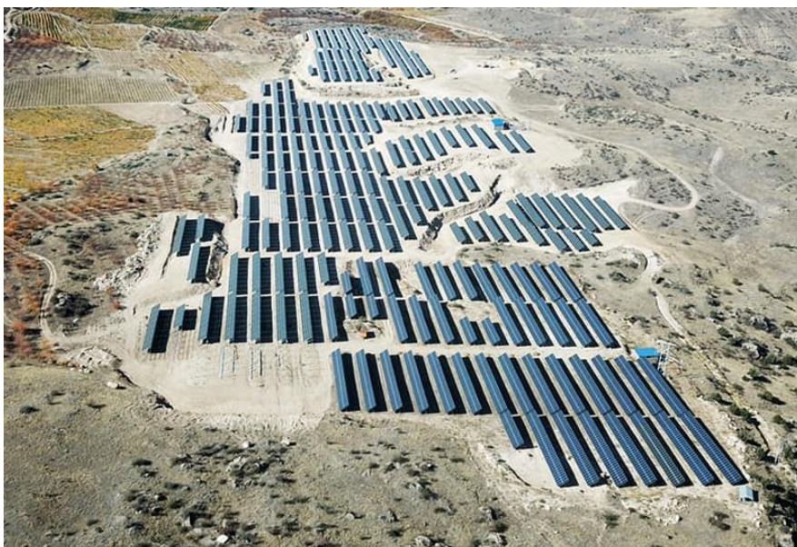
Figure 2. The largest solar PV plant with capacity 5.2 MW was put into operation in Armenia in October 2020 by Optimum Energy LLC and connected to grid. (Photo by Optimum Energy)
