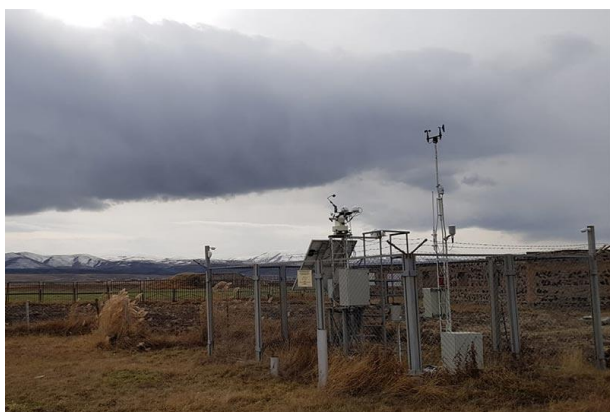
Figure 1. Meteo station for Masrik-1 solar PV station.
